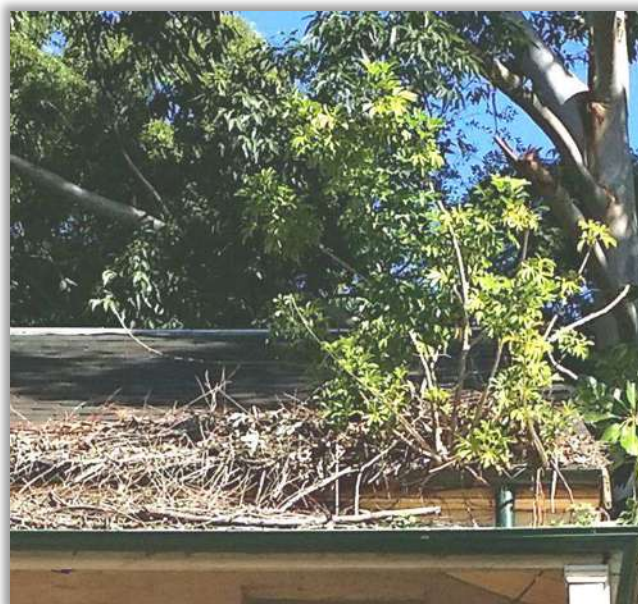
A plant growing in the guttering on the top floor of a property in Mt Vernon St; note the collapsed gutter. (Image: V. Simpson-Young)
