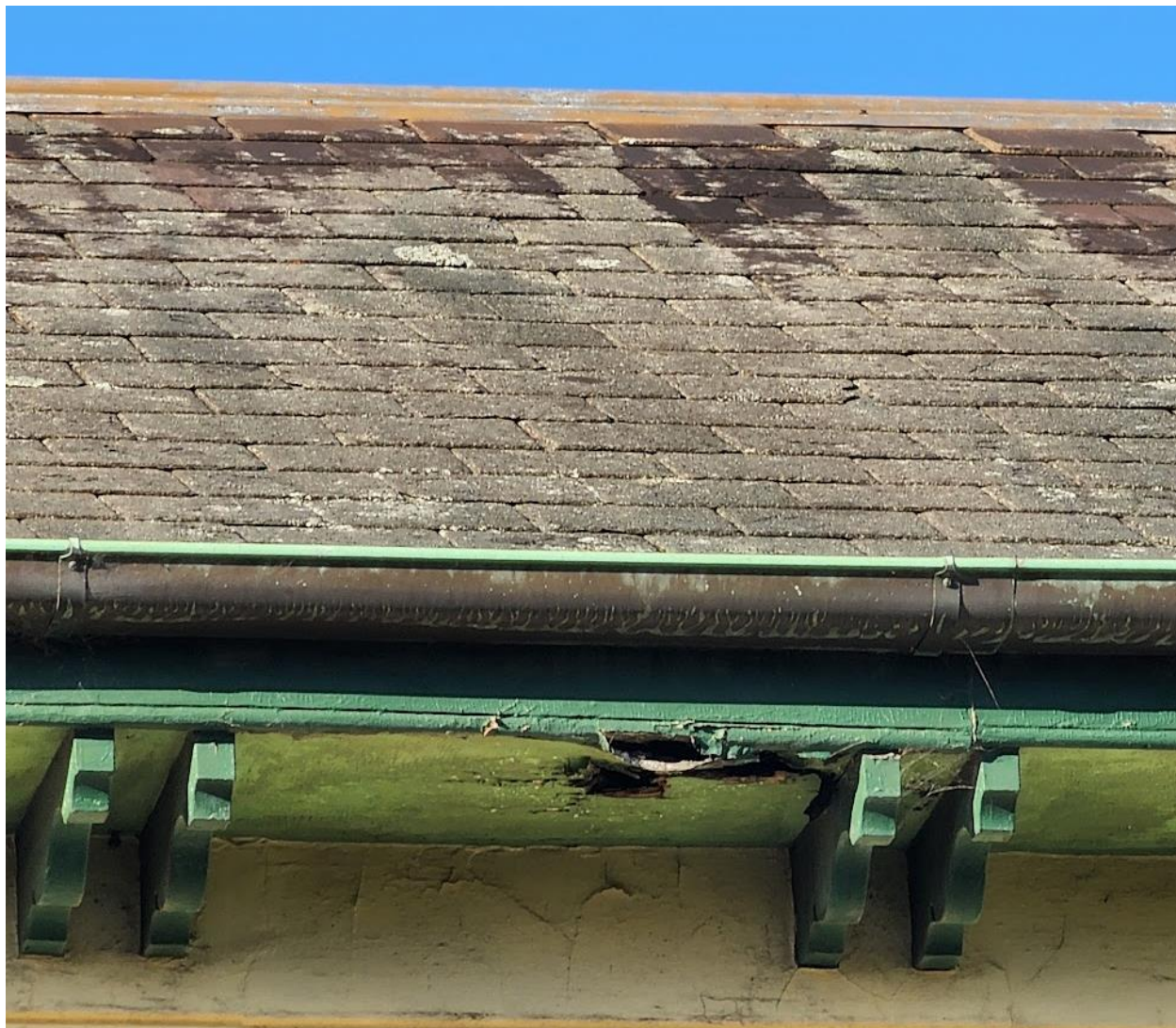
Figure 2 The soffit of the eaves is deteriorating
