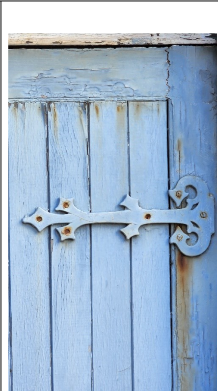
Figure 4 A detail of one of the original hinges
