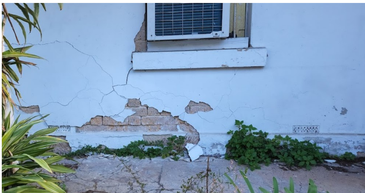
Figure 5 Number 22 Forest Street, June 2023 showing cracking which appears to have been caused by the impact of a heavy object
