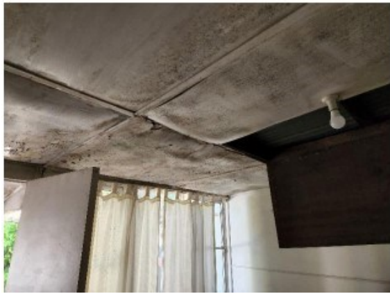
Figure 8 This image in the Structural Report of a water damaged ceiling is in the skillion of number 20 not the main house
