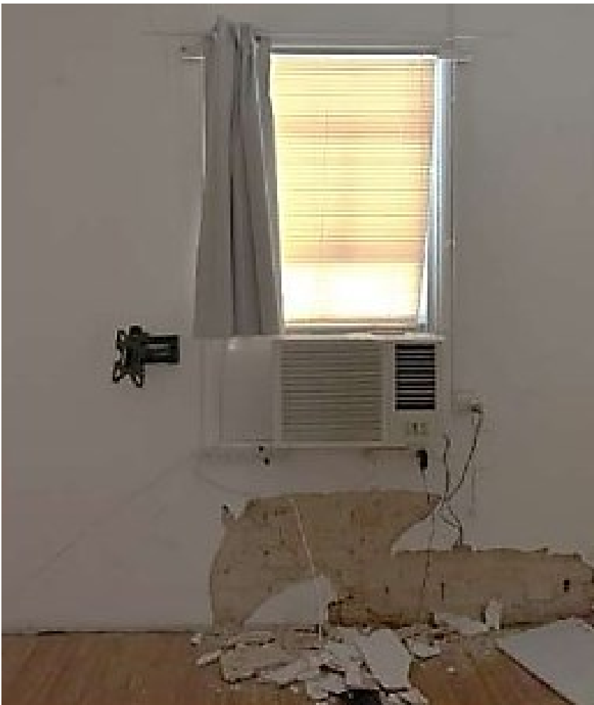
Figure 7 Inside view of the north eastern wall of number 22, Weir Phillips Heritage Impact Statement 20—22 Forest Street Forest Lodge , March 2023.. The wall beneath the window appears to have been impacted by a heavy force
