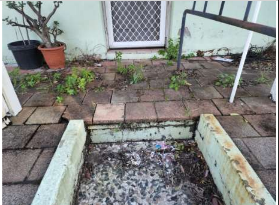
Figure 28 The level of the front garden has been raised to the height of the veranda. This with leaking gutters and downpipes is likely to exacerbate damp.
