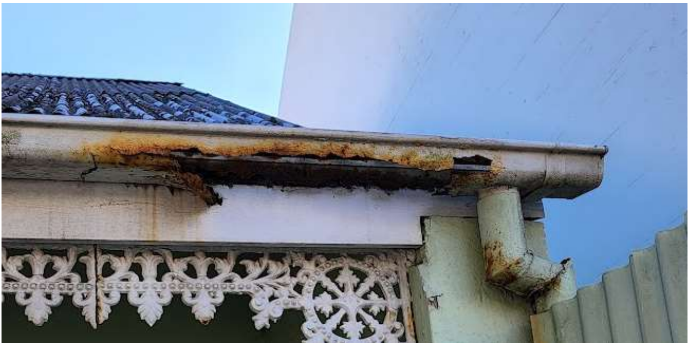
Figure 23a The guttering is in poor condition
