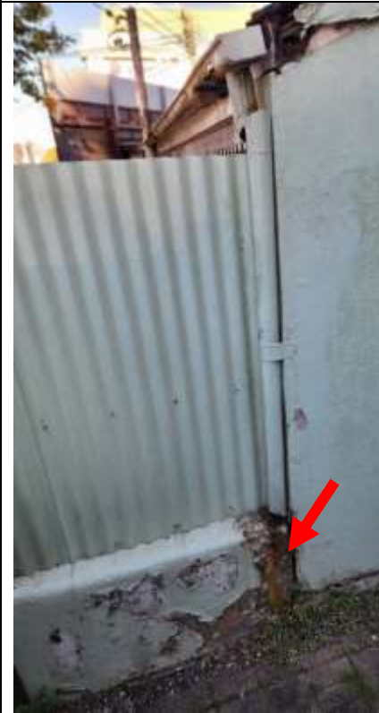
Figure 23 The crack can be attributed to a leaking down pipe. It should be noted that the palisade wall fence is not rotating but remains in the vertical. The problem could be ameliorated by fixing the down pipe and removing the paving next to the wall
