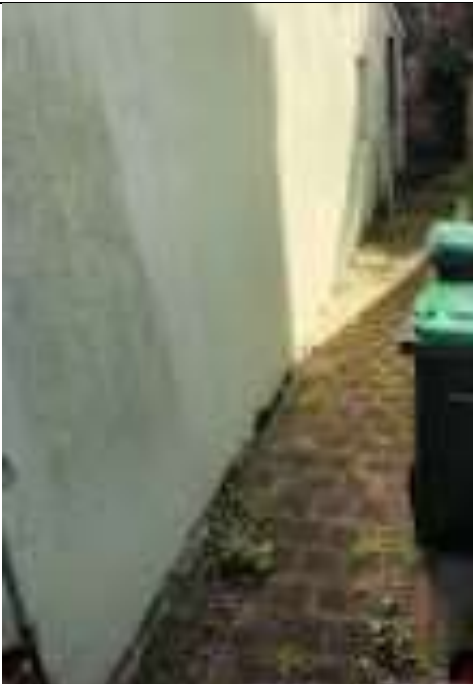
Figure 27 Hard paving has been constructed right up to the eastern wall of the house
