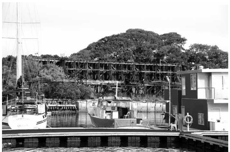
The ruined coal bunker viewed from the Fish Market. This is one of the foreshore sites approved for development which should have the CRG planning principles applied before final development approval is granted. Photo: Bruce Davis
